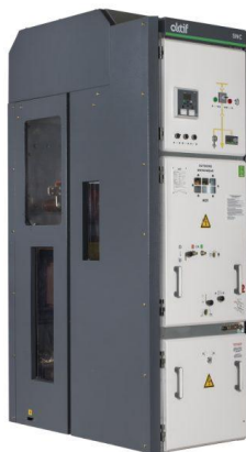
Figure 2 Metal switchyard [AKTIF].
