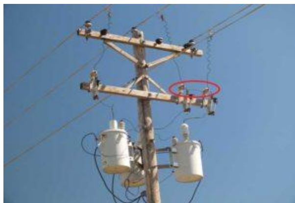
Figure 2 Lightning Arrester [Daws on Power].
