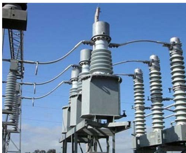
Figure 1 Installation current transformer [Google].
