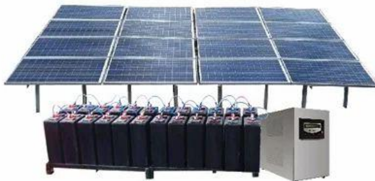
Figure 4 Off grid solar panel [IndiaMart].
