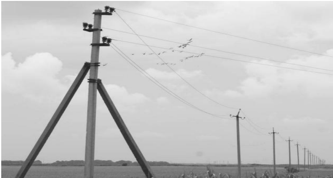
Fig. 1 Supports of 6-10 kV overhead lines in open areas (farmland).
